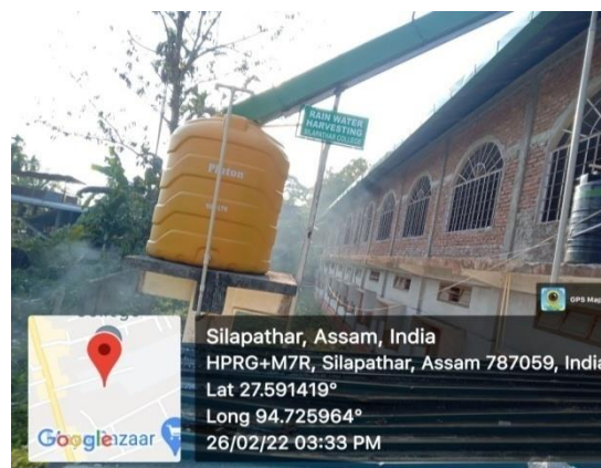
At Arts Departmental Block (Ladies toilet)
